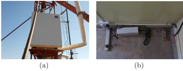
Figure 5: Our equipment in Macha: (a) the base station and (b) the power supply.
